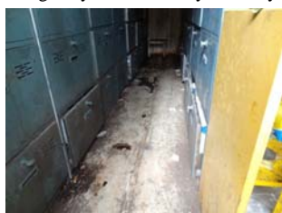
圖 6: 廢液貯存室地板破洞 Corroded floor inside the storage chamber
